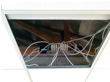
A TeroLight unit in situ
